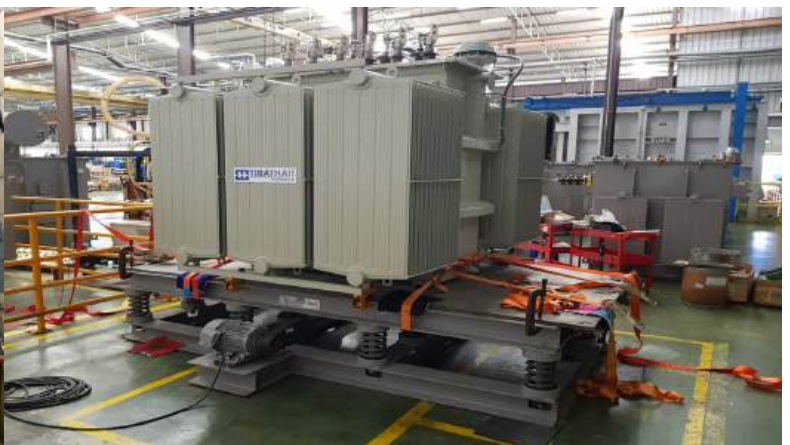
Vibration Proof Transformer
