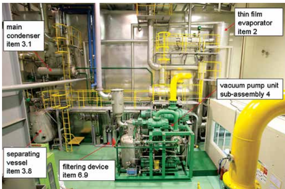
Fig. 6. Vapour phase drying equipment with thin film evaporator designed by Hedrich vacuum system, Germany
