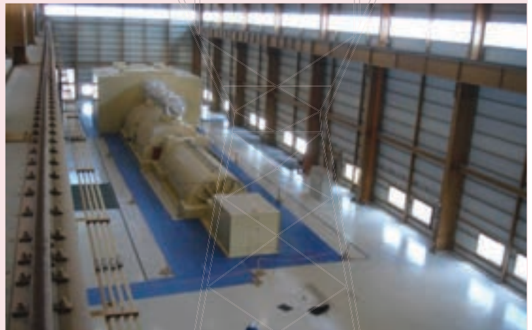
Figure 4 : Steam Turbine & Generator
